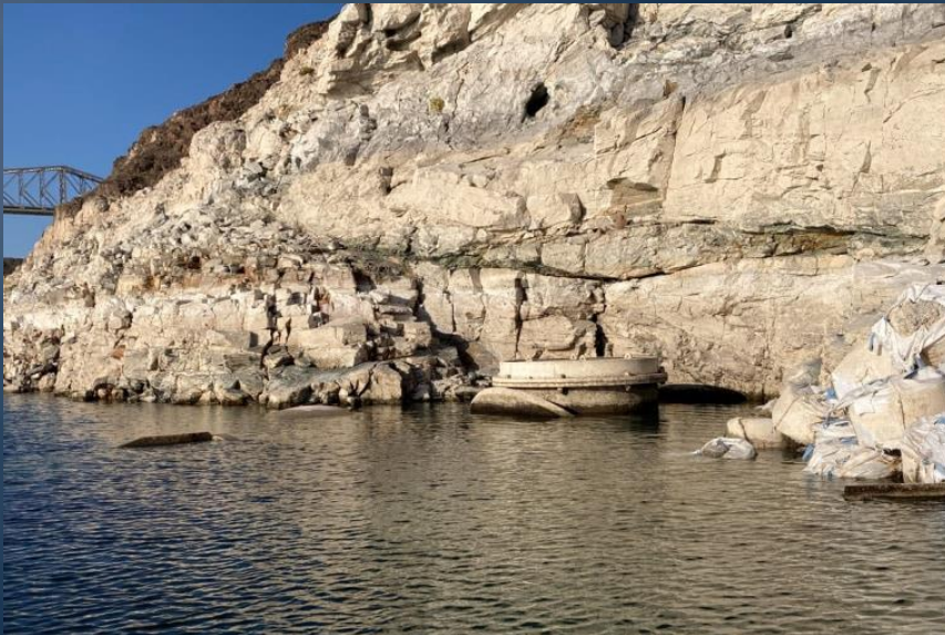
SNWA's Original Intake
